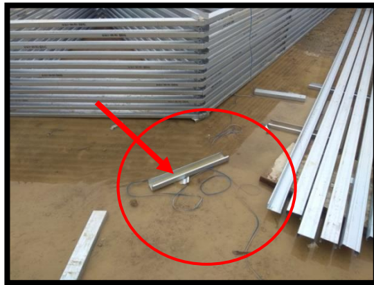
Figure 5. Submerged cable Source: Personal Documentation
