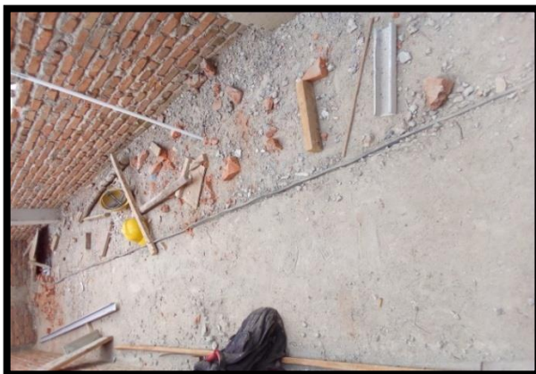
Figure 23 . Rubber Anti Earthquake ( dilatasi / joint f Iller )
