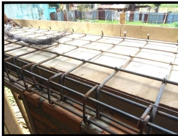
Figure 8 . Canopy Plate Reinforcement
